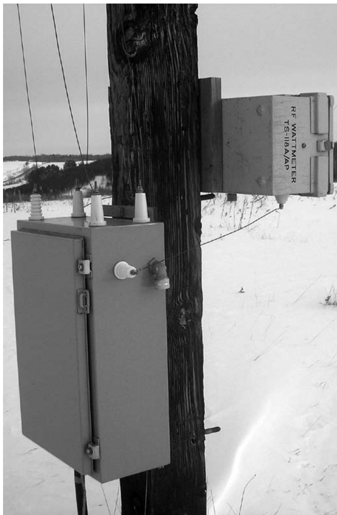
Figure 6 — Balun (left) and terminating resistor, mounted below the center of a rhombic for direction switching
