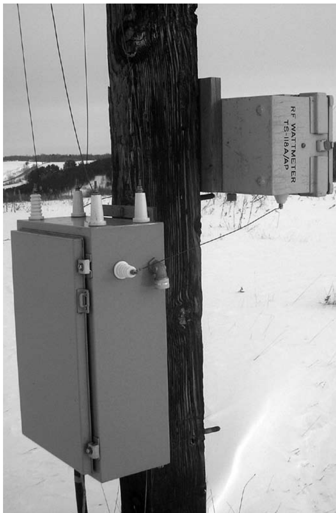
Figure 6 — Balun (left) and terminating resistor, mounted below the center of a rhombic for direction switching
