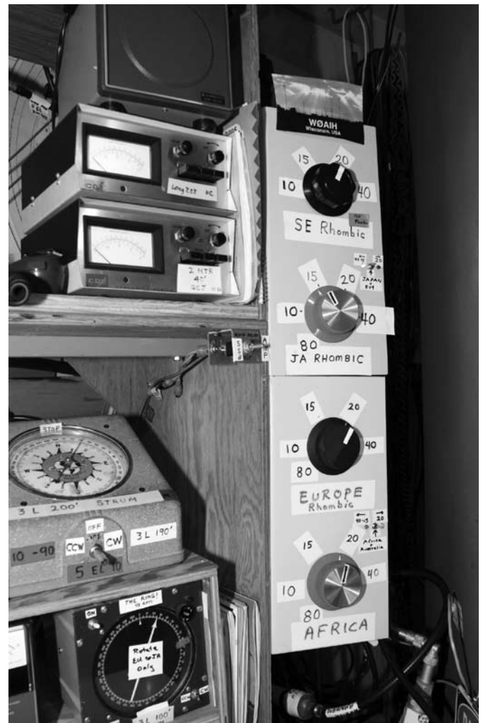
Figure 7 — Switches in “the chalet” direct rhombics to each operating position.
