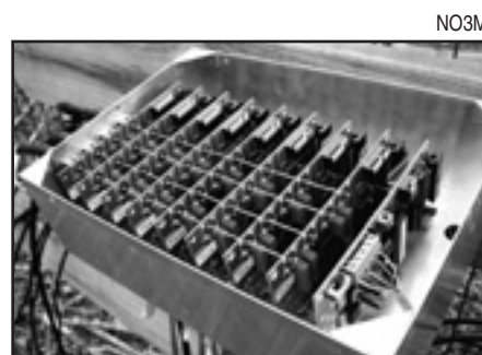
Figure 2 — Antenna switching matrix in its enclosure: Radio ports at the top are wired in parallel. The microprocessor board is in front.
