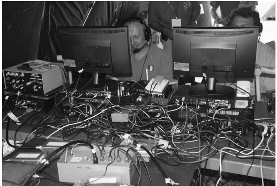
Figure 2 — All that filtering and switching didn’t necessarily make for the tidiest arrangements at R33A (ES5TV and ES2RR), which placed second).
