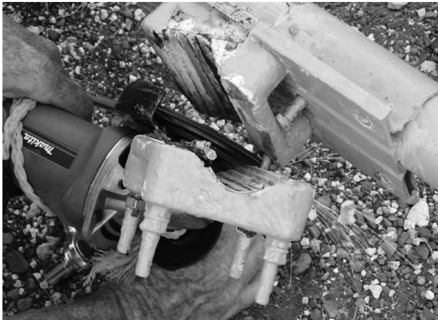
Figure 4 — Cutting apart totally fused stainless bolts and a Hy-Gain boom-to-mast mount. We had to do this to five similar assemblies at PJ2T in order to get them off the towers.
