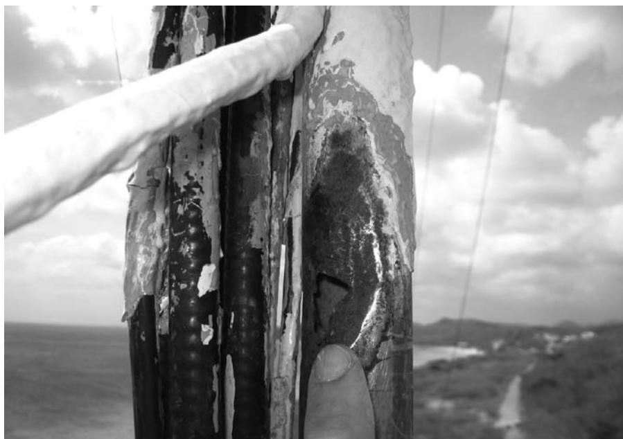
Figure 3 — March 2010: A horrifying hole in a Rohn 55 tower leg that we almost missed. This section was nearly new in 2000 when it was installed. The leg was 100 percent good a few inches above and below the hole.
