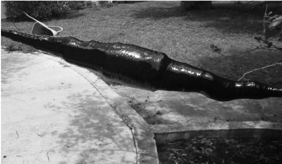
Figure 6 — This joint between Phillystran and a quarter-inch EHS guy wire tail contains a large egg insulator. All parts have been painted with epoxy, totally encapsulated in duct seal putty, wrapped in Scotch 33 tape and varnished.
