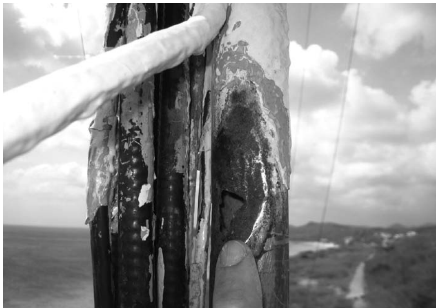
Figure 3 — March 2010: A horrifying hole in a Rohn 55 tower leg that we almost missed. This section was nearly new in 2000 when it was installed. The leg was 100 percent good a few inches above and below the hole.
